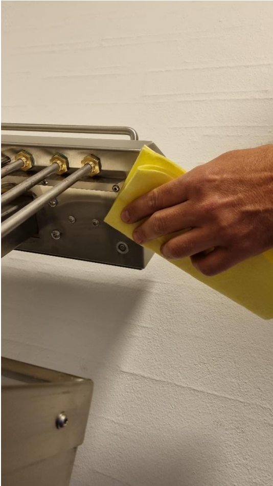
Exercise particular caution in the area near the magnetic contact. Regular cleaning is particularly important here.
